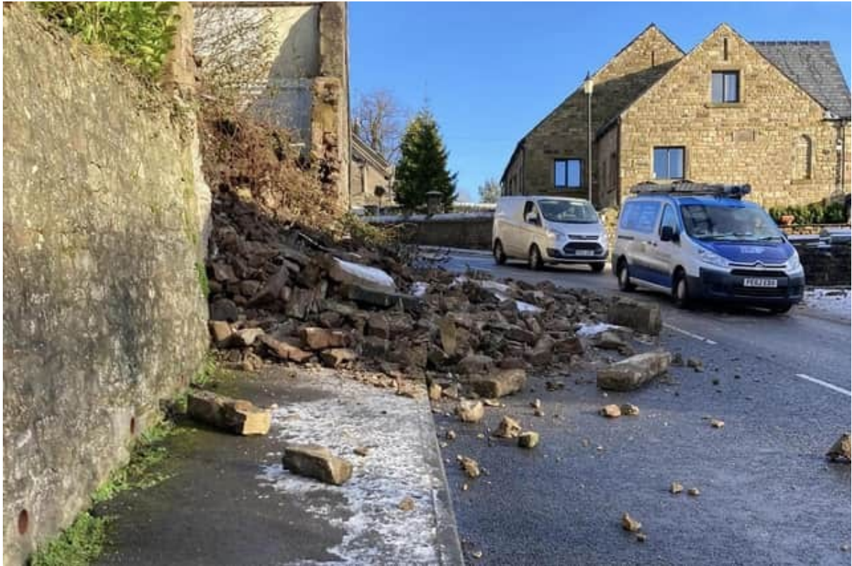
This photo taken by Eric Filbin from The Red Door Cafe shows the collapsed building in Church Brow
